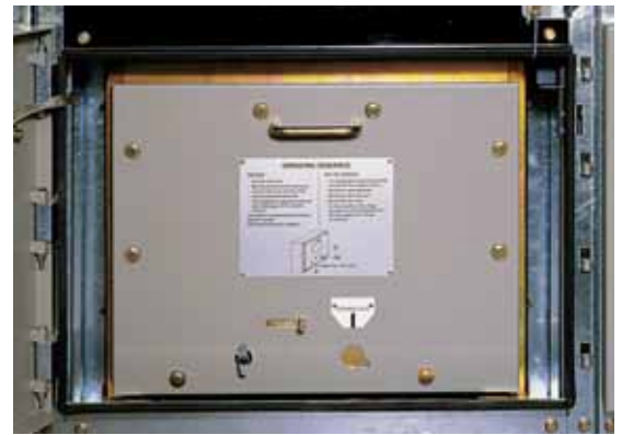
Compartment with withdrawable voltage transformers.
