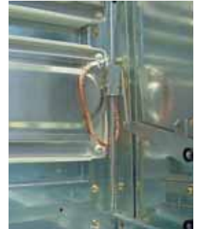
Detail of metallic shutter earthing.
