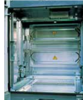
Metallic segregation shutters of the contacts.
